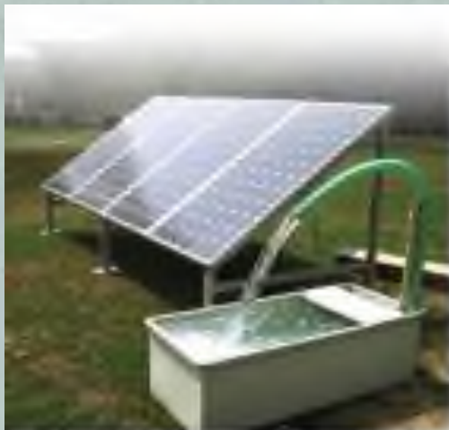
PV-powered pumping system
