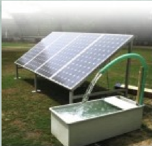
PV-powered pumping system
