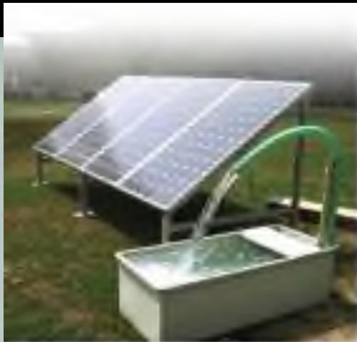
PV-powered pumping system
